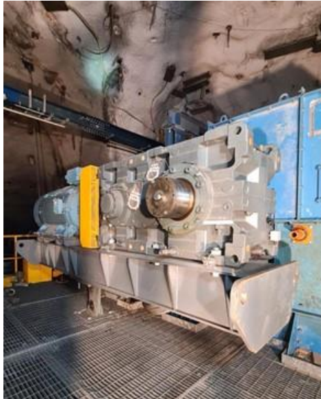
Transfer tower gearbox assembly
