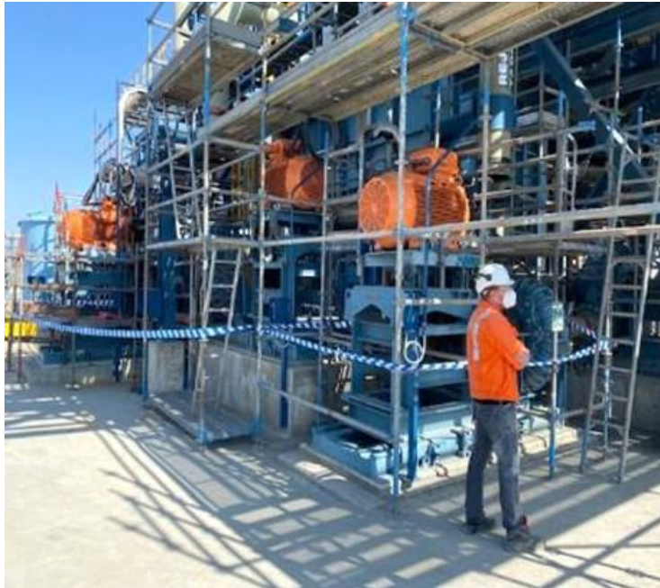
Cyclone energization and cold commissioning
