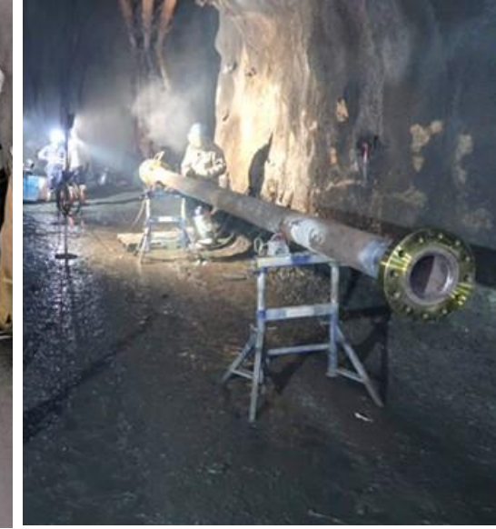
Mechanical and piping reticulation system
