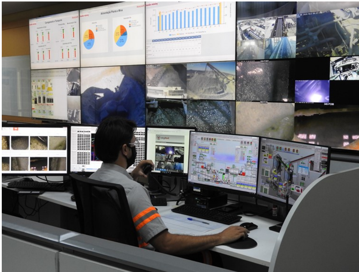
Chapada mine and mill control room
