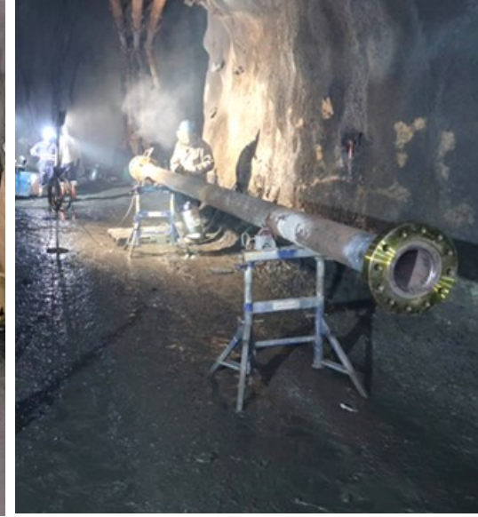
Mechanical and piping reticulation system
