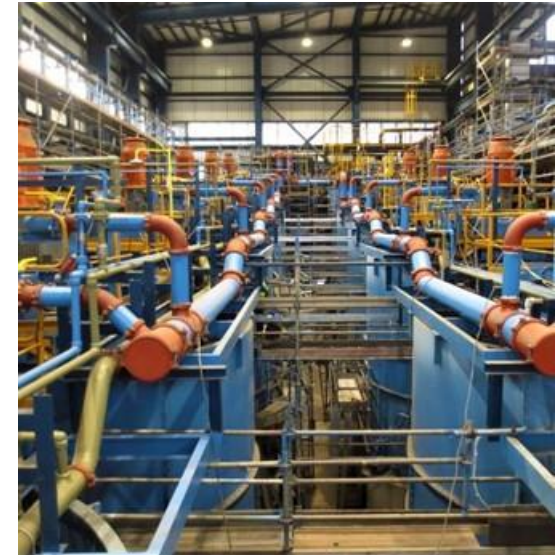
Flotation building piping
