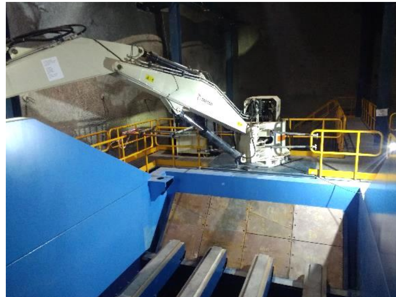
Crusher chamber – rock breaker and hopper
