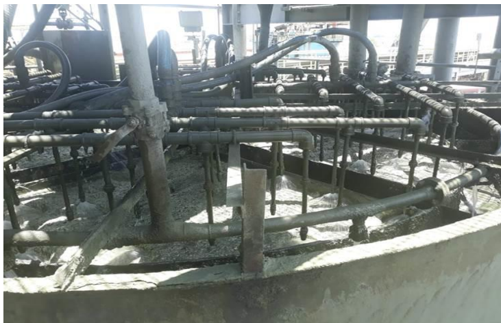
Column flotation circuit
