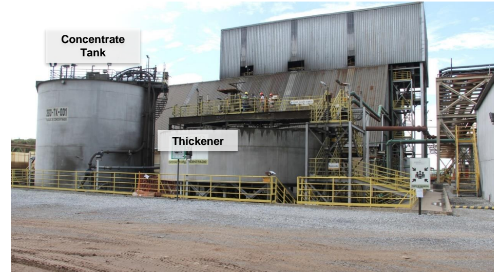
Concentrate tank and thickener
