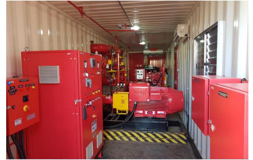
Fire pumping system
