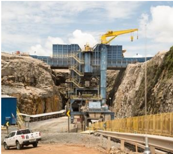
In-pit gyratory crusher
