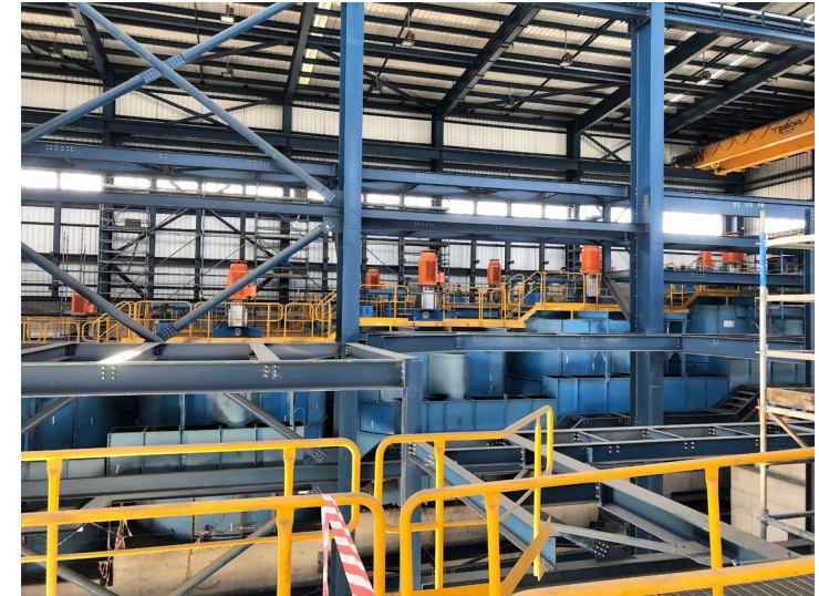
Flotation cells in new zinc plant building
