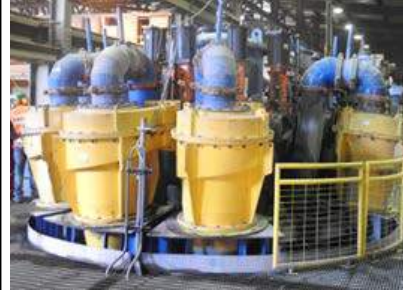
Cyclones & Feed Pumps
